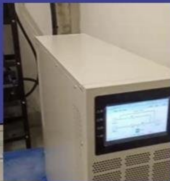
60kwh lithium batteries
