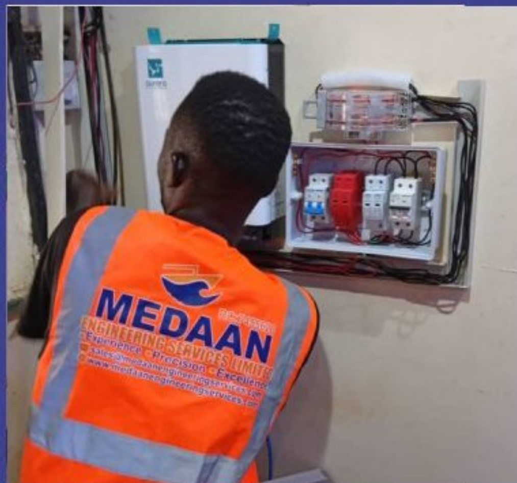
Backup system battery pack project
