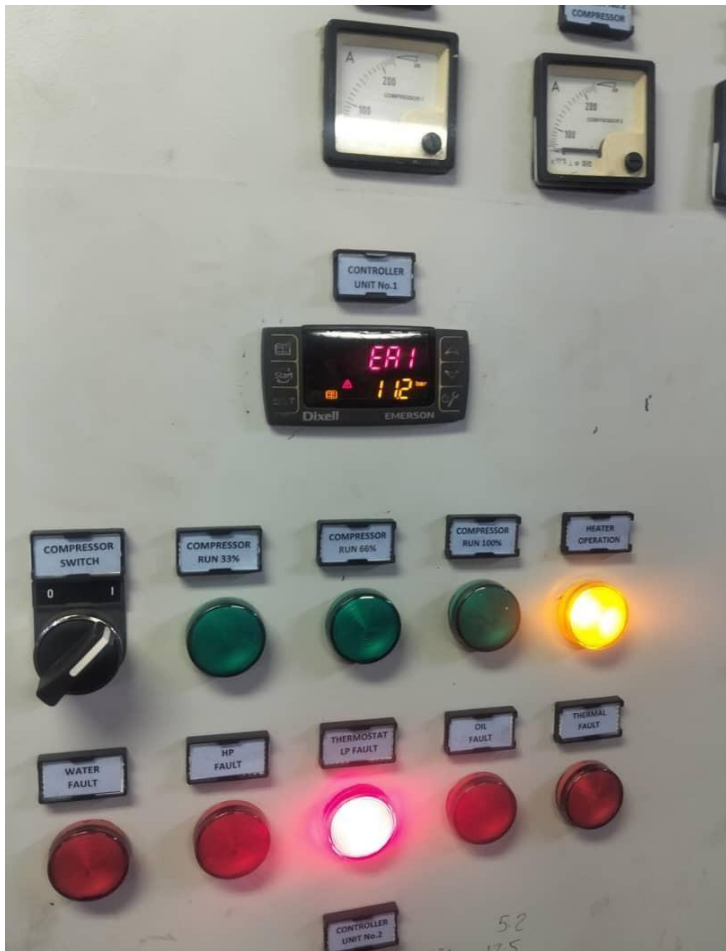
Low Pressure Alarm System Before Repairs
