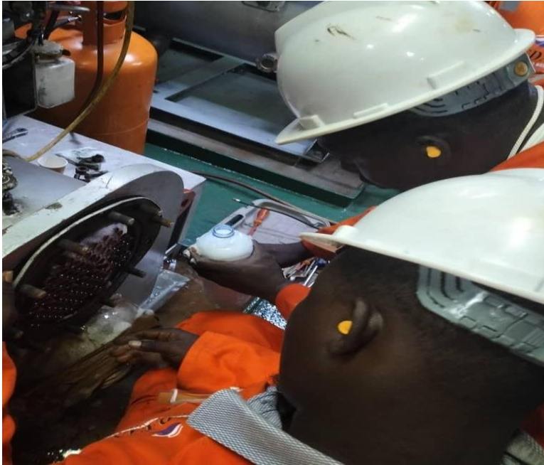
A.C condenser leakage findings
